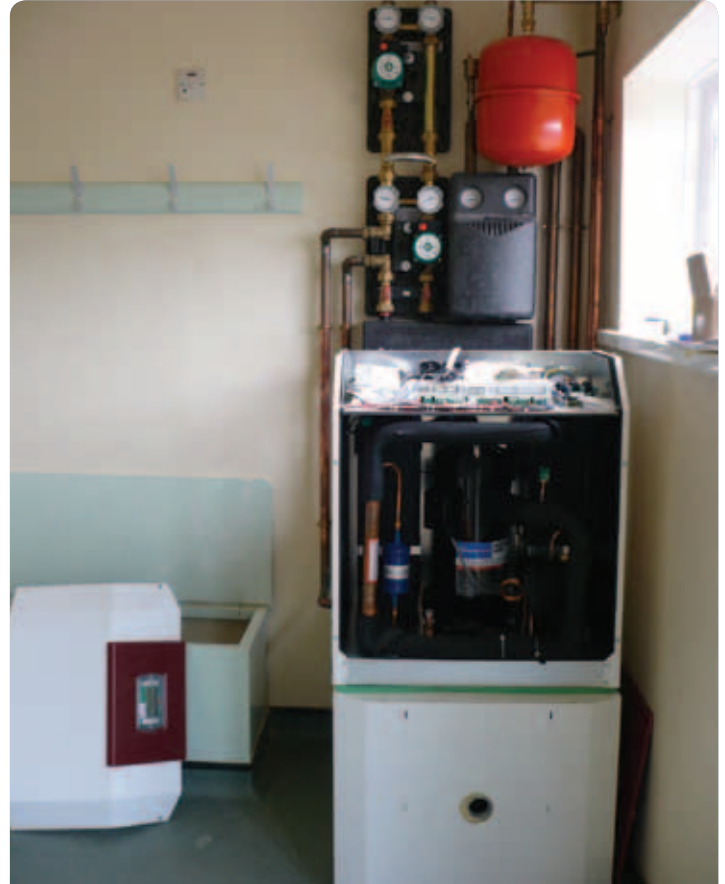
Installed heat pump
