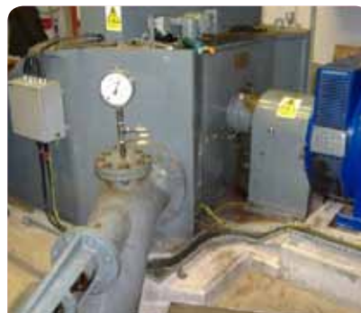
Plant room of a 500 kW hydro scheme in Cumbria
