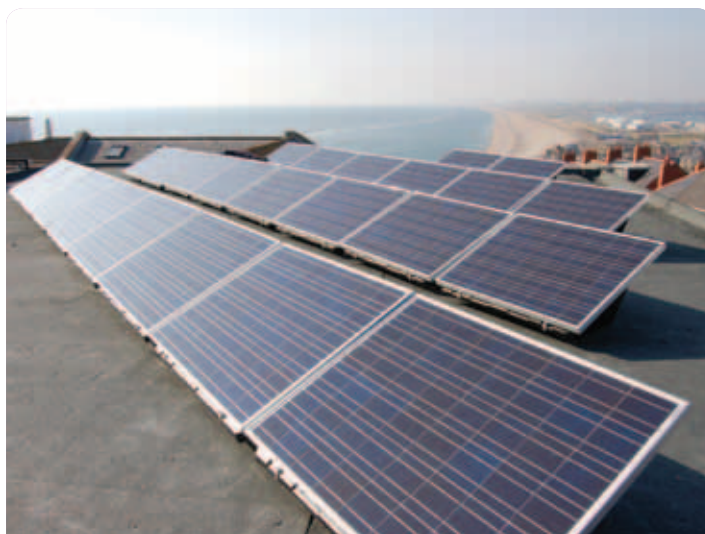
Solar PV at Underhill Primary School, Portland
