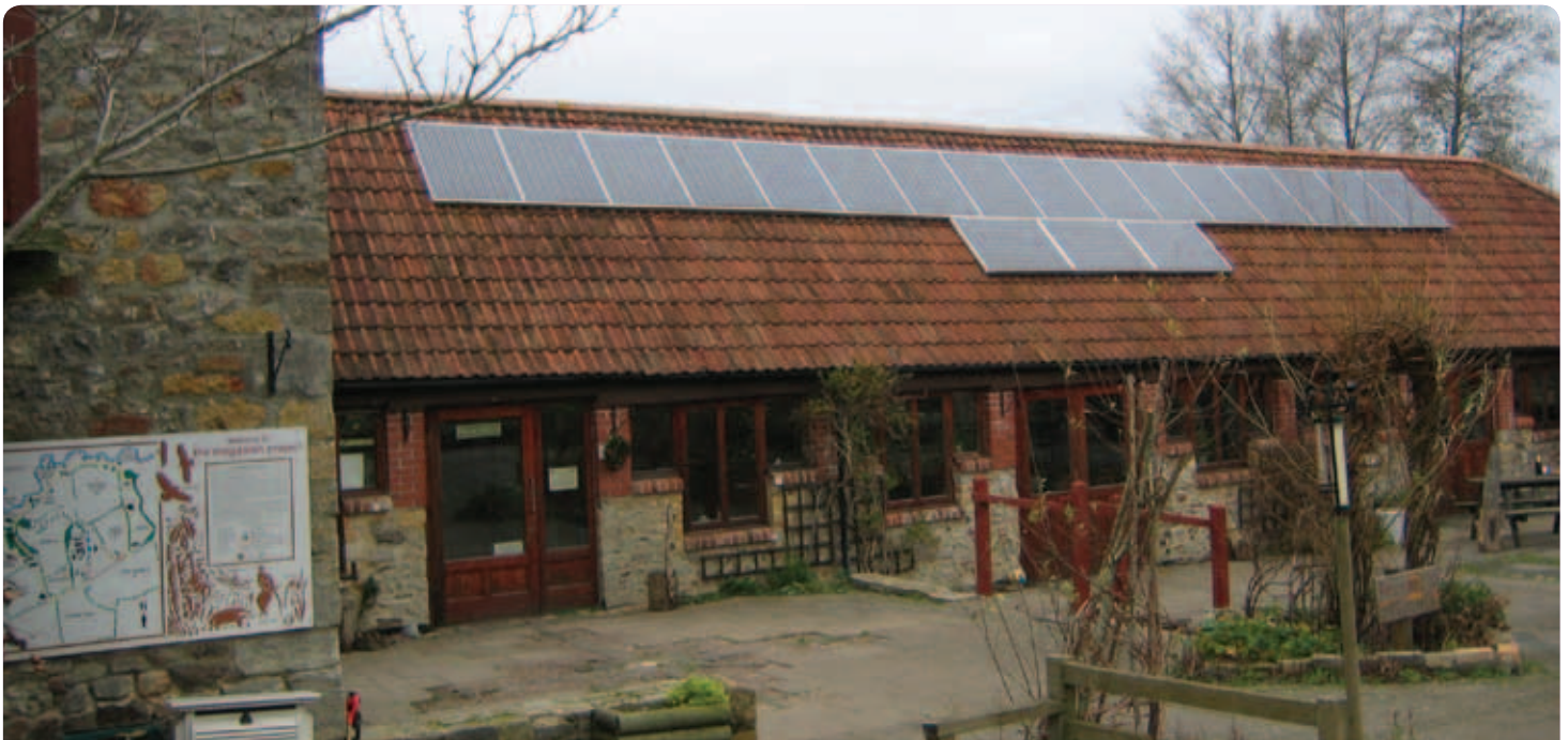
Solar PV roof panels at the Magdalen project, Dorset
