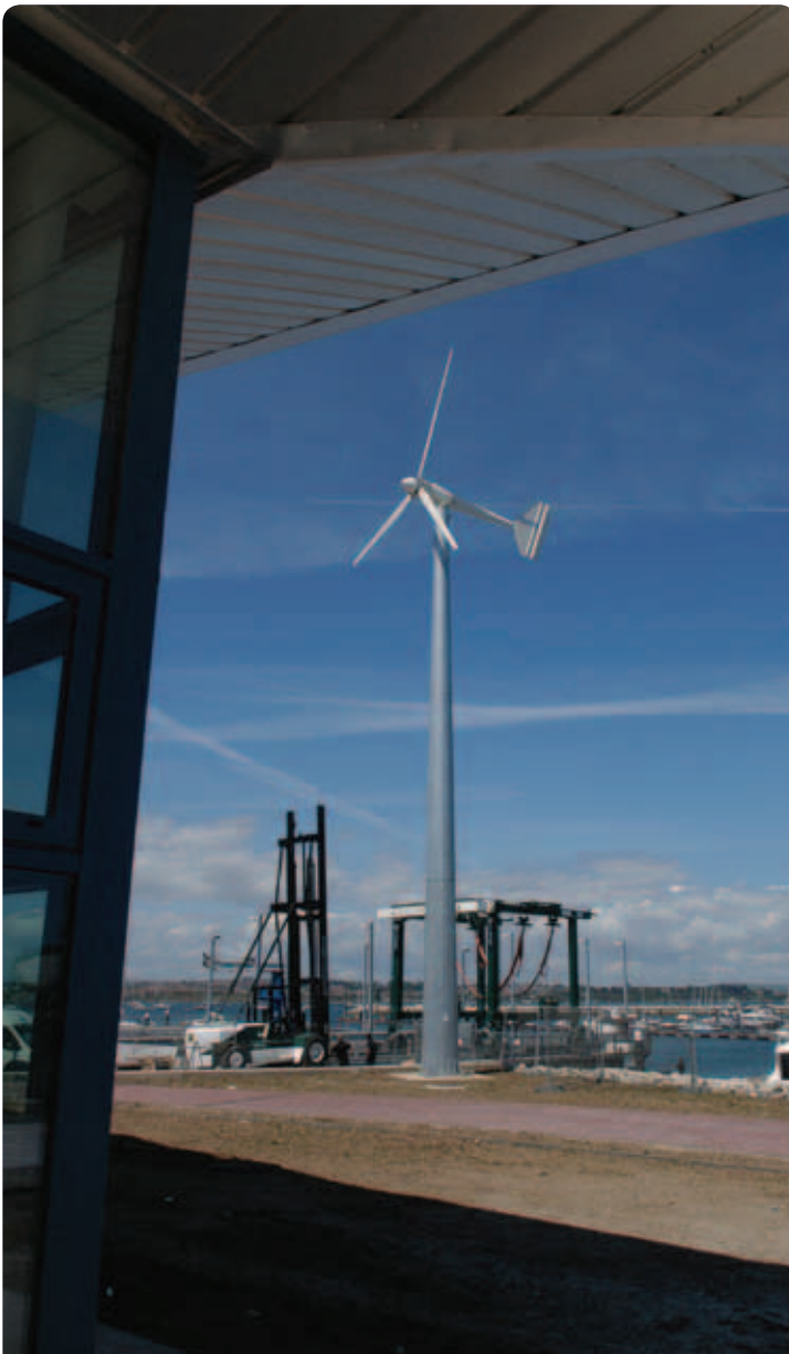
20kW wind turbine Portland Marina
