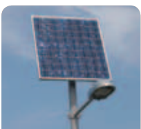
Solar power street light
