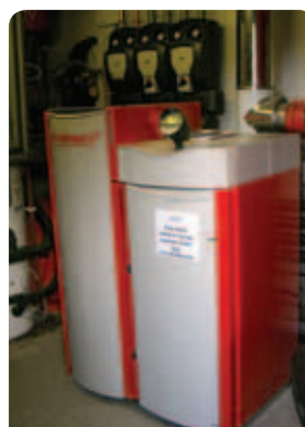
50kW pellet boiler Kingcombe Centre, Dorset
