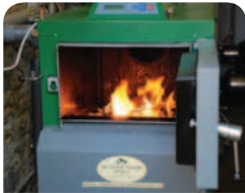
25kW log boiler Mapperton Estate, Dorset
